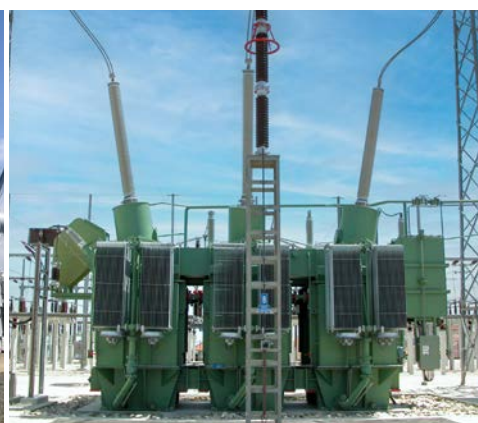
Three-Phase Transformer 170MVA, 400kV (Portugal)
