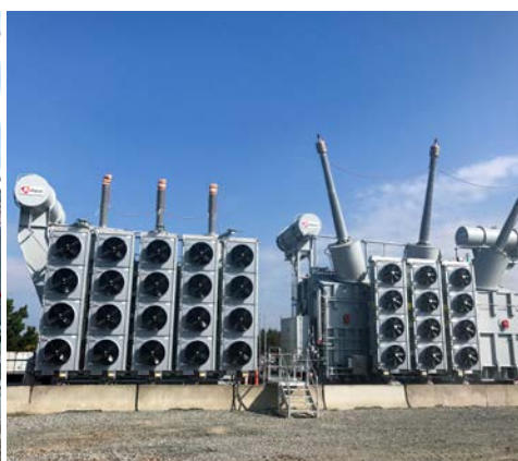
Three-Phase Autotransformer 760MVA, 230kV + 750MVA, 525kV (USA)
