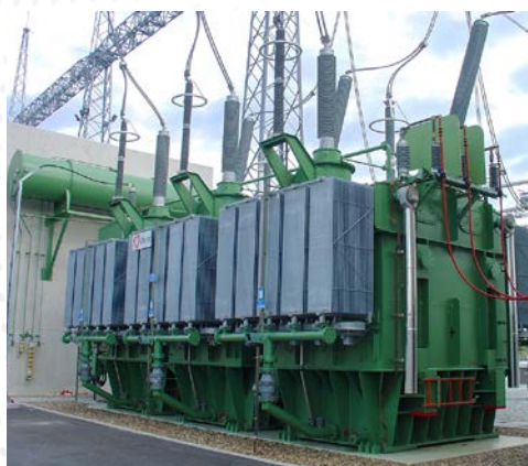
Three-Phase Autotransformer 450MVA, 400kV (Portugal)
