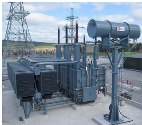
Three-Phase Autotransformer 1200MVA , 400kV (UK – Scotland)
